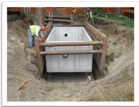
New Winooski East Master Meter Vault
