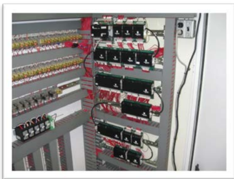
Continued upgrades to SCADA RTUs at remote sites and at the Treatment Plant.
