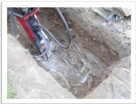
At Lawrence Heights in Jericho a hydraulic hammer being used to explore the extent of ledge rock in advance of the project design for the water main replacement.
