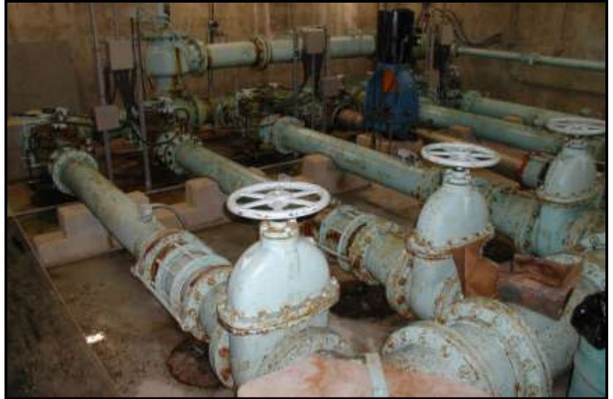
Williston North Pump Station Rehab (before)
