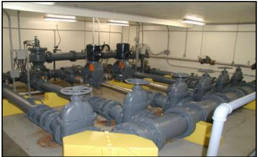
Williston North Pump Station Rehab (after)
