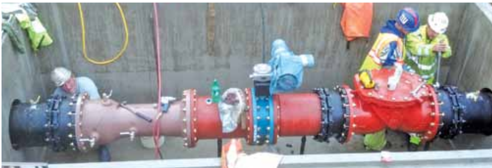
Relocation of Williston North meter vault as part of construction of the High Service Cross-tie Project
