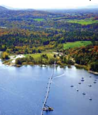
Assembling concrete anchors onto 42" diameter south intake at staging area in Shelburne Bay Park (2007)
